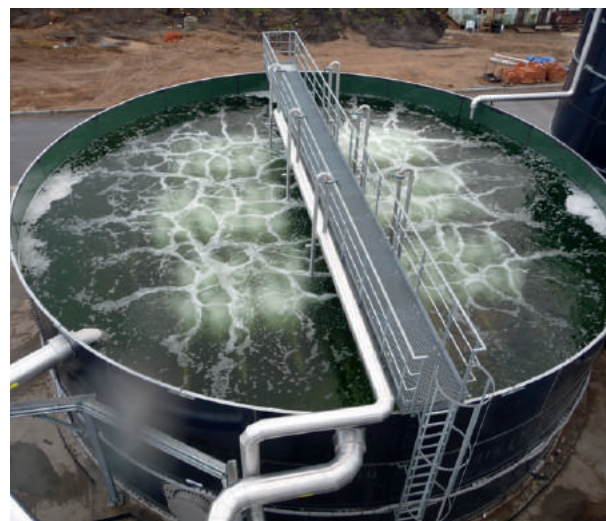
Industrial wastewater being treated in an open reactor.
